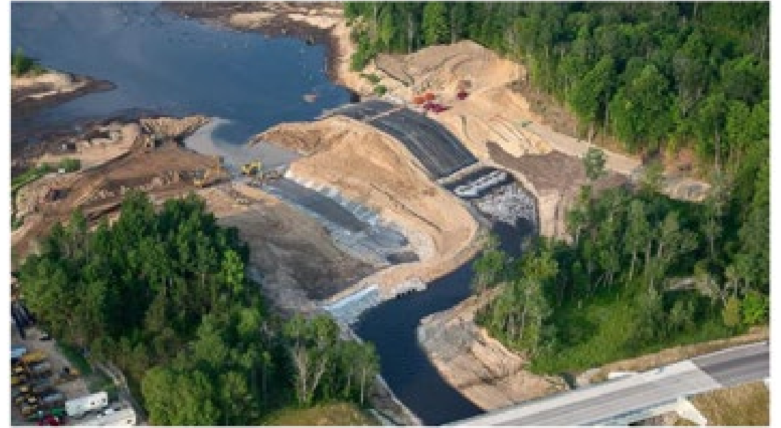
Boardman River Dams Ecosystem Restoration Project (dam removal, Traverse City, Michigan) ( https://www.lre.usace.army.mil/Media/Images/igphoto/2002067168/ )
